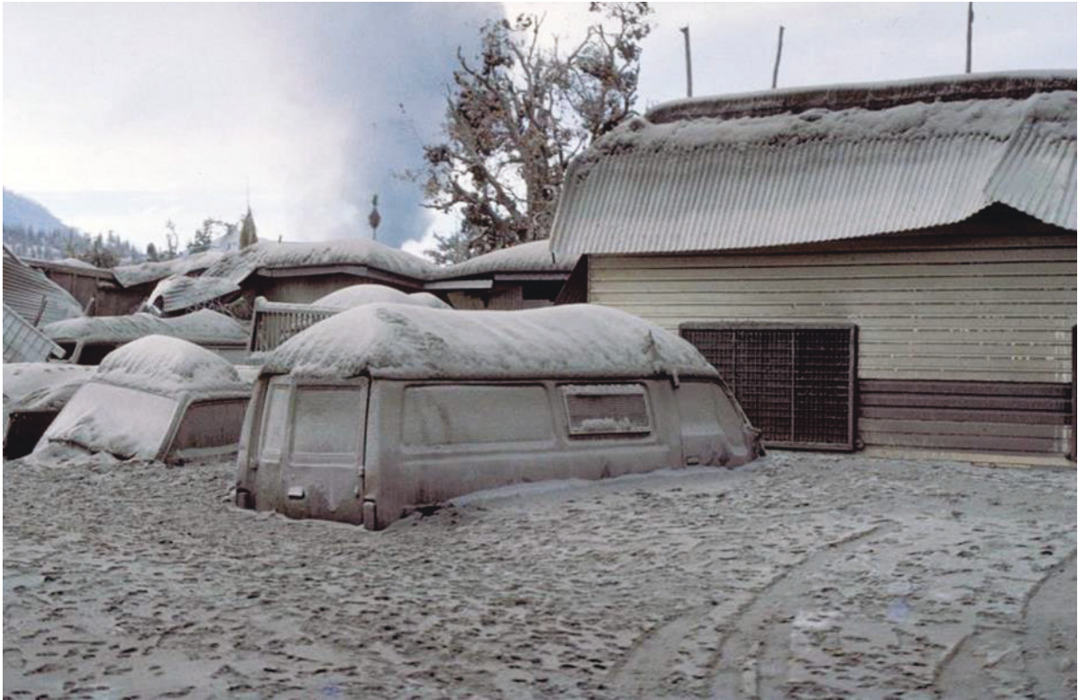
Figure 2.12: Effects of Volcanic Deposition on A Roof
