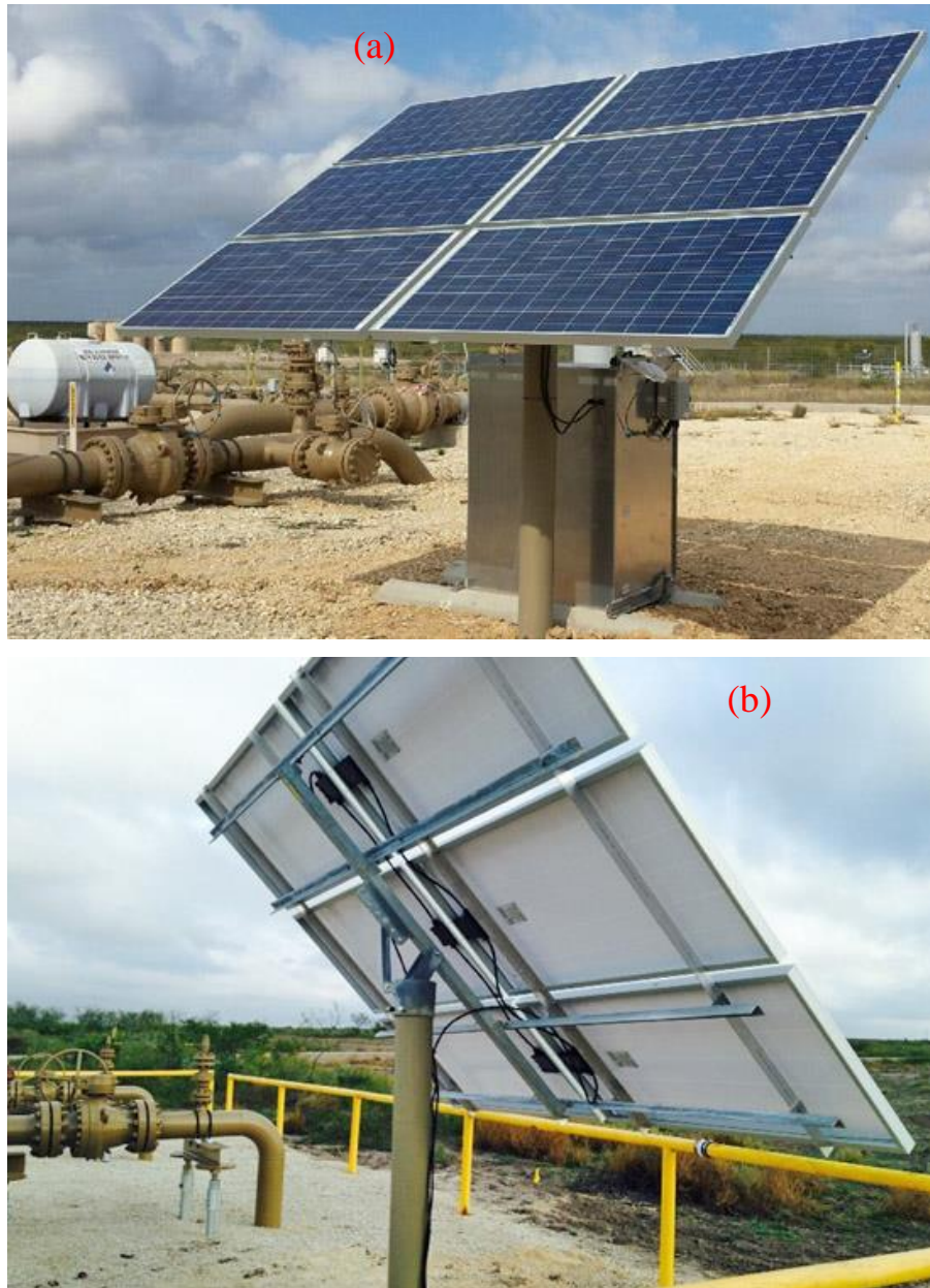
Fig. 7. Practical application of solar PV powered cathodic protection CP, (a) front view with batteries and controller, (b) back view of solar PV (SPCP 2021).
